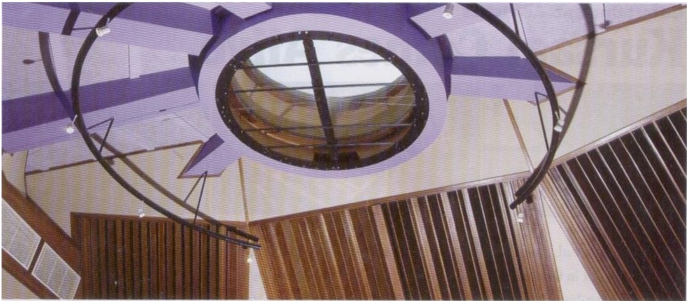
A controllable sky light opening in the centre of the ceiling offering natural daylight or complete darkness to the room
