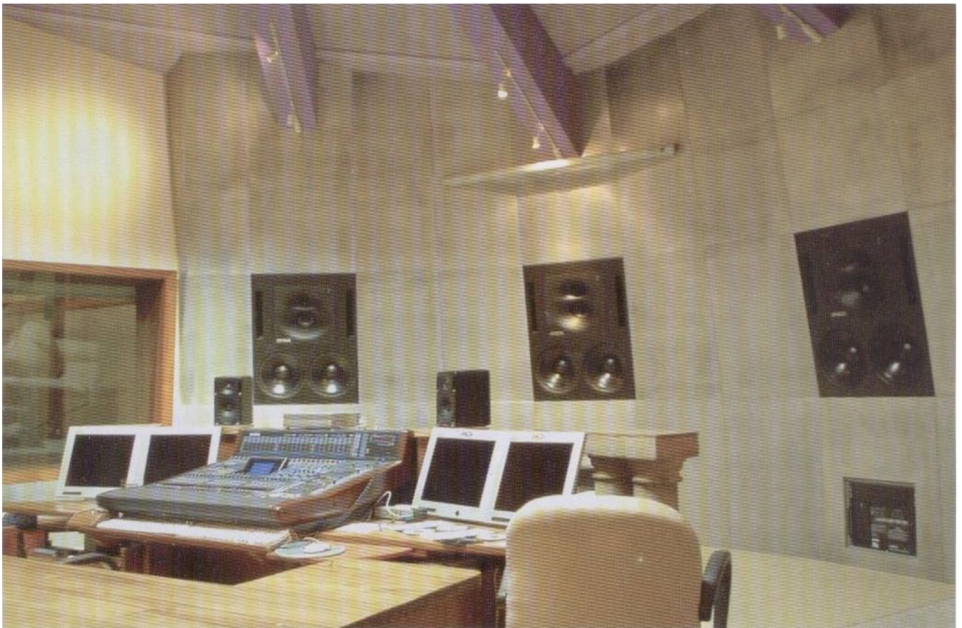
Front wall covered with aluminum giving this control room a sci-fi and very grand feeling
